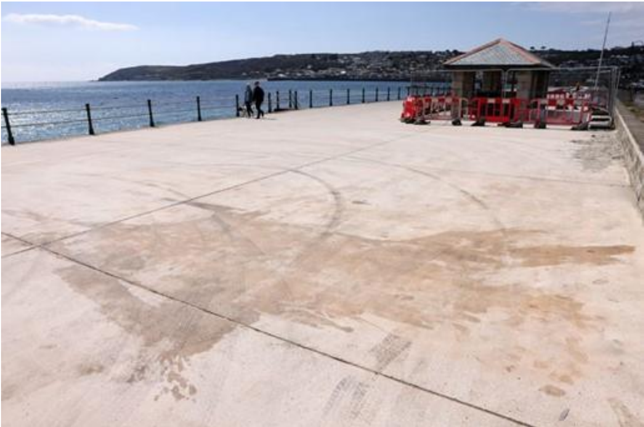
Staining prior to cleaning process
