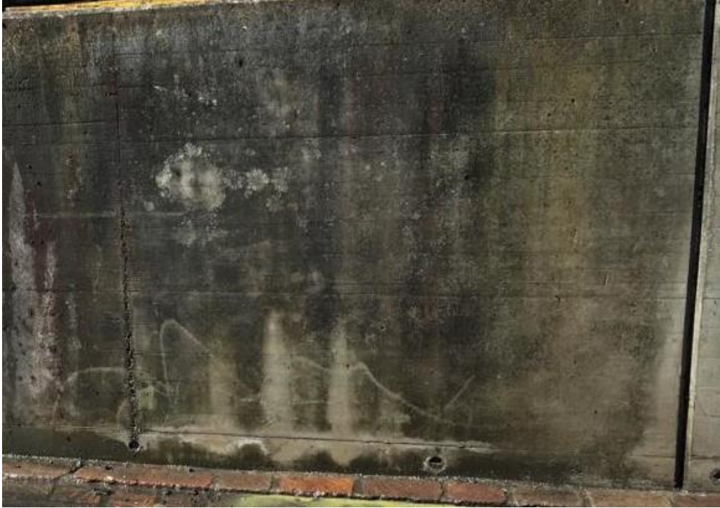
Concrete Wall: Very dirty
